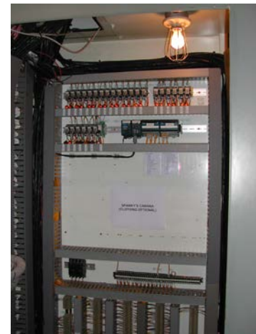
Figure 2 Upgraded Control System
