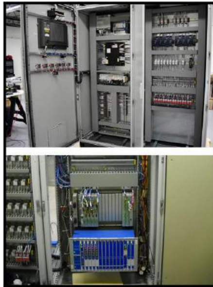
Interior of New Control Cabinet
