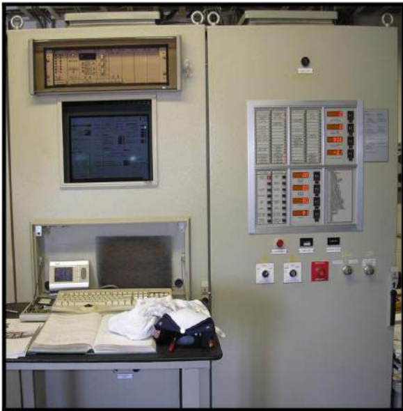
Original System On-Site
