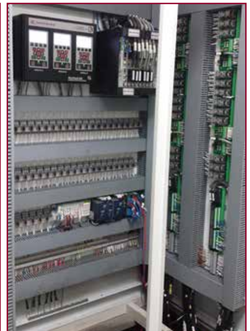
Interior of New Control Cabinet
