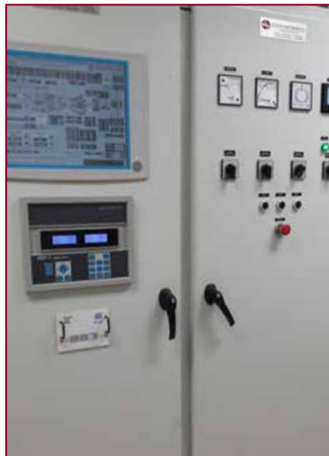
New System Installed
